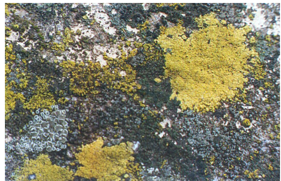
Lichens growing on concrete
