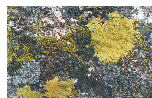
Lichens growing on concrete
